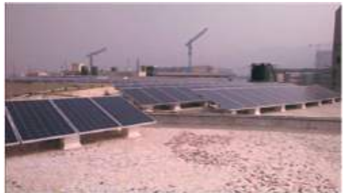
Photograph of solar plant installed at SIES Nerul
